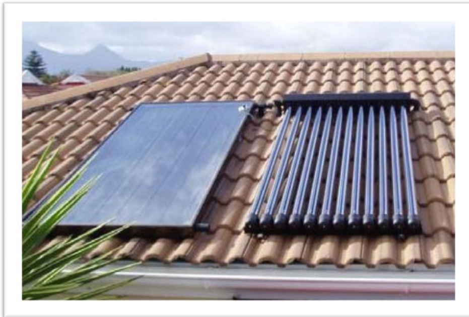
Two types of solar thermal panel
