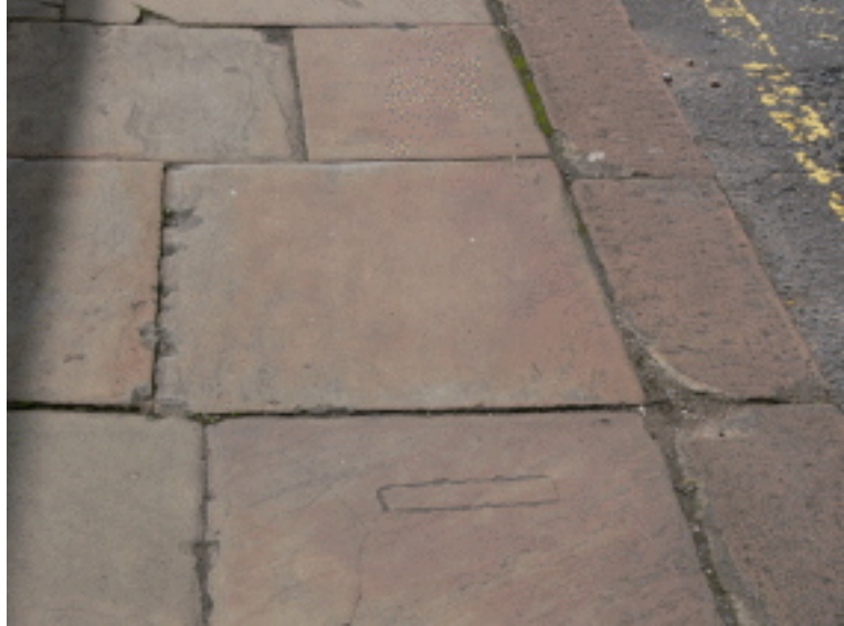
Picture 3.2 Original stone flag paving
