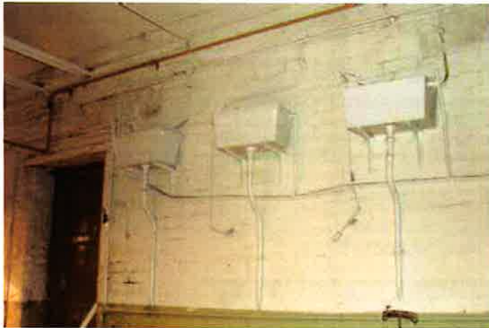
027 – Cisterns, Queens Street Mill, Briercliffe, Burnley
