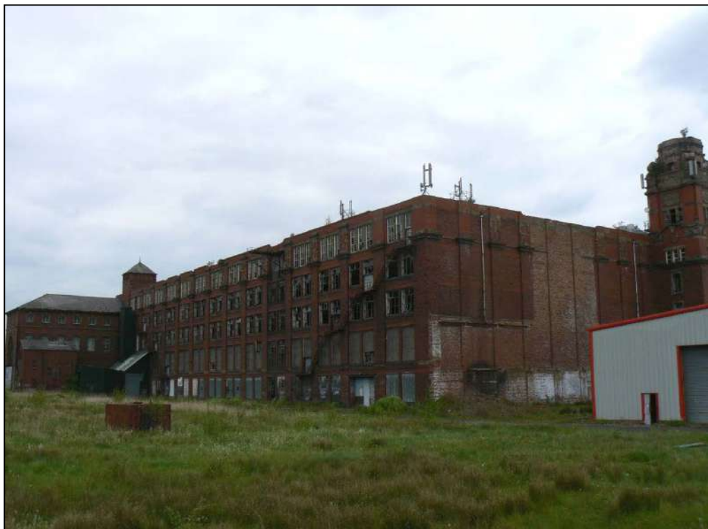
Plate 10: The derelict spinning block and engine house at Wesley Street Mill in Bamber Bridge
