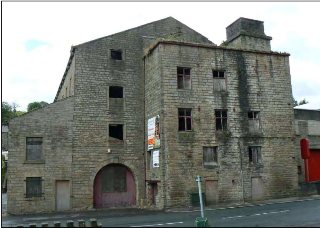
Plate 21: The derelict Grade II-listed Waterside Mill in Bacup
