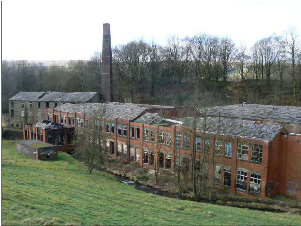
Plate 23: The unoccupied Eden Wood Mill in Edenfield, which was in very bad condition in 2012. Dating originally to 1796-1806, the mill was expanded in the early twentieth century
